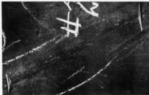
Fig. 7—Deep seam which did not fail at pressure of 10,500 psi.: 7-in.-o.d., 23-lb., N-80 casing.
